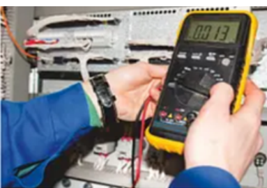
Low Voltage Systems
