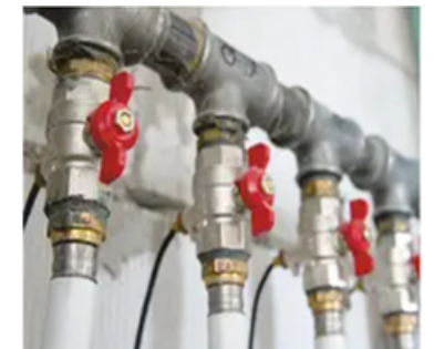
Water Supply Control
